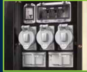
Convenience sockets provide power directly from the generator
